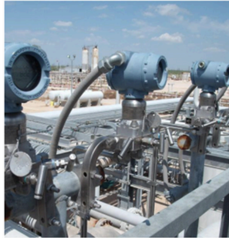
New field transmitters for the driven compressors
