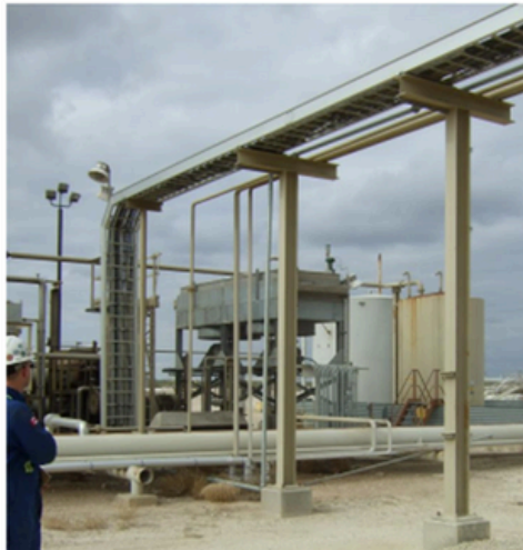
Newly installed cable raceways
